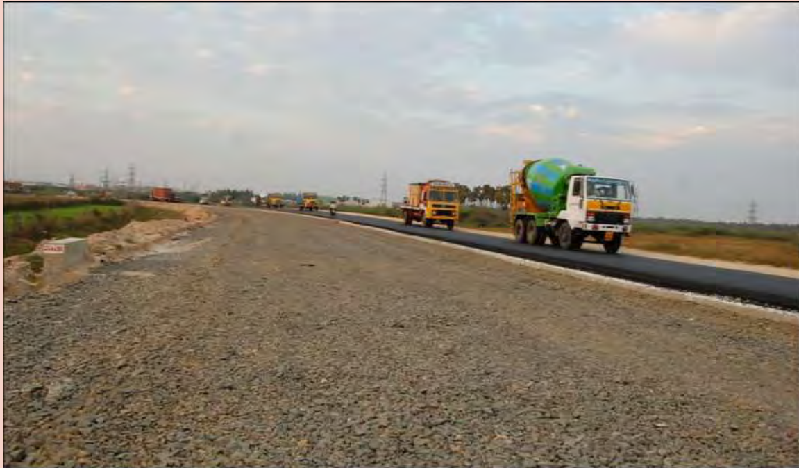
Ongoing Bypass work at Pondhur near Sriperumpudur under the Industrial Corridor Project.
