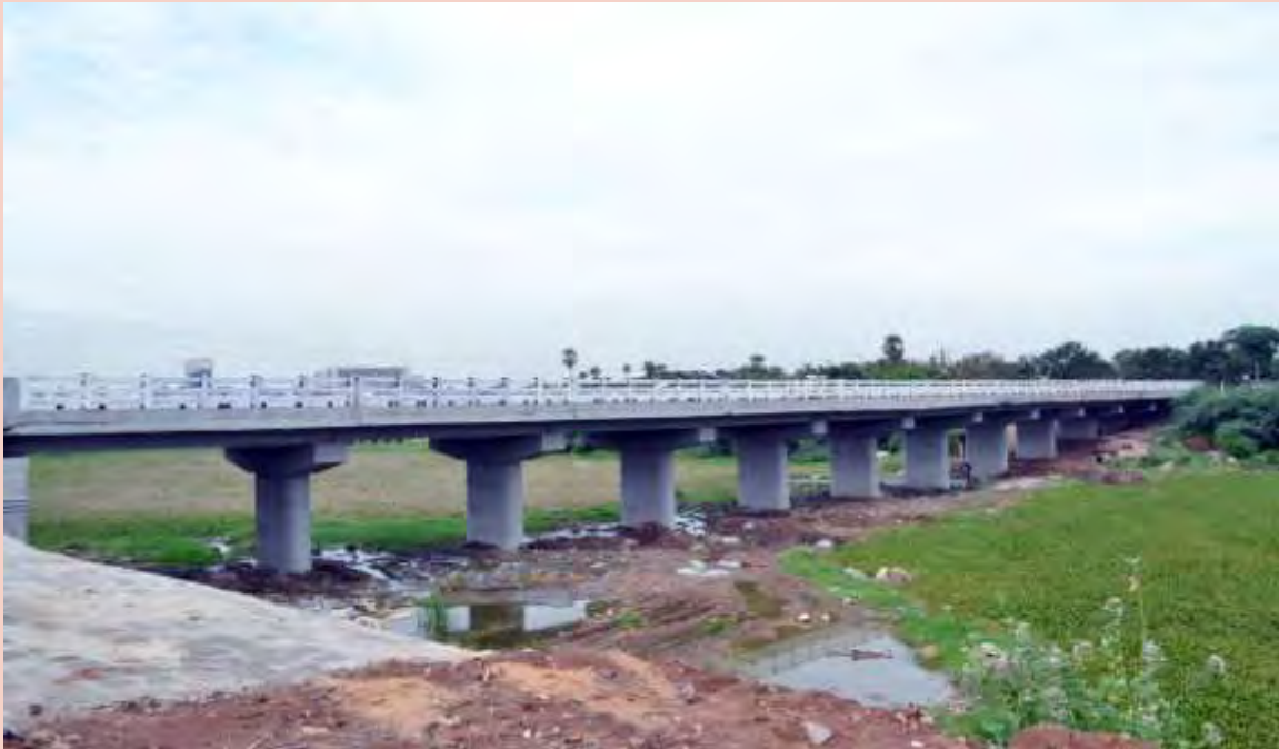
Bridge across Adyar at Nandambakkam, Chennai inaugurated by the Hon'ble Chief Minister on 09.10.2012
