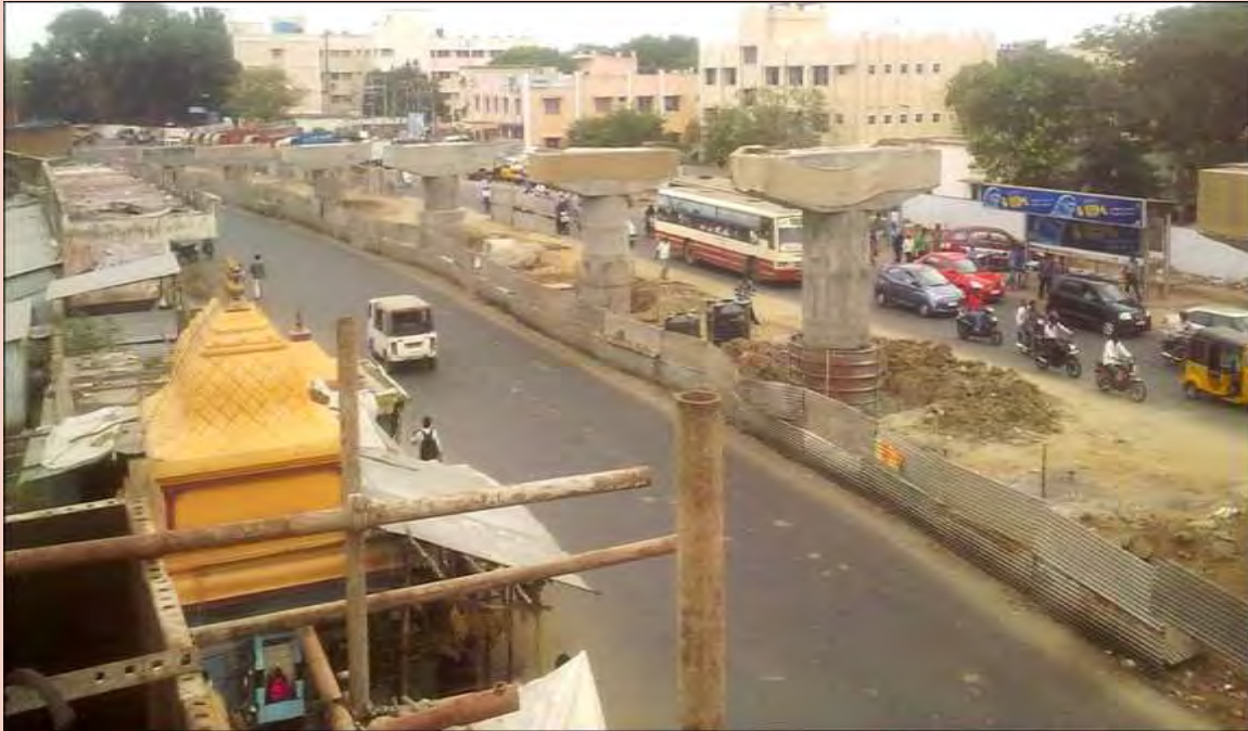
Ongoing Grade Separator work at the Nelson Manickam Road junction, Aminjikarai, Chennai.
